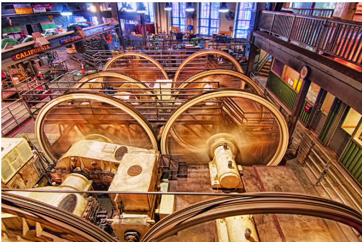
Cable Car Power
